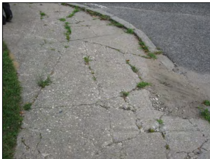
Photograph No. 4: View of deteriorated sidewalk/curb area at Union Avenue and Mill Road.
