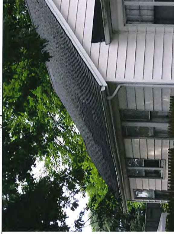
View of roof deterioration.
