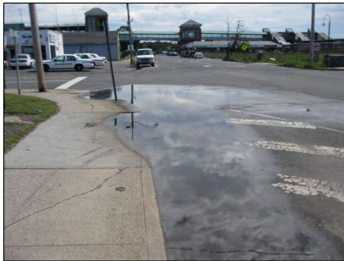
Photograph No. 5: View of pooling water along Railroad Avenue.
