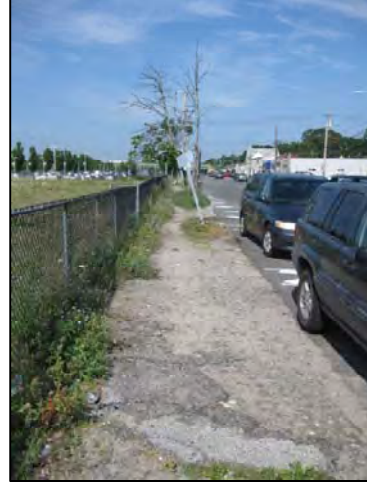
Photograph 8: View of deteriorated sidewalk areas along Railroad Avenue.
