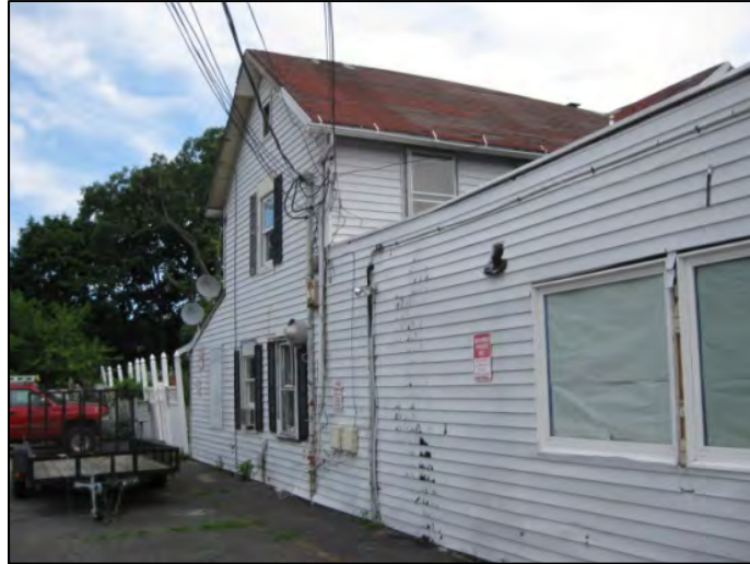
Photograph No. 3: View of a deteriorated mixed-use commercial and residential structure along Garrity Avenue.
