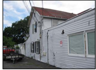
Photograph 2: View of deteriorated building along the east side of Garrity Avenue
